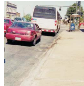
Rutting at Bus Stop.
