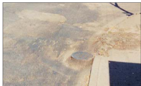
Failed Catch Basin.
