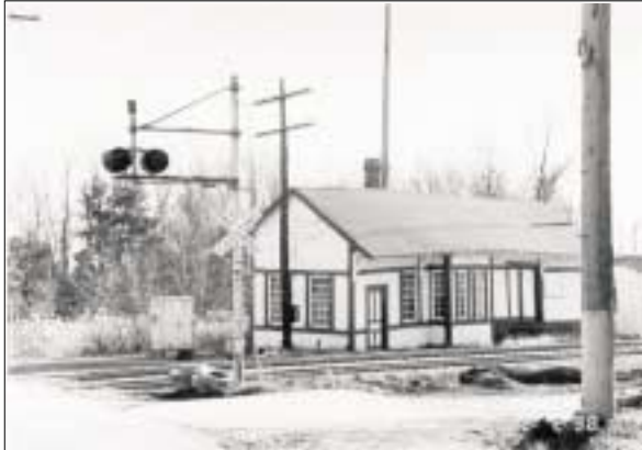
The historic Falls Junction train depot is in need of repair. Plans to move and rehabilitate the structure into a museum and to run train excursions can serve as the foundation for improving the center of town.
