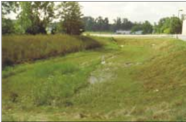
Inadequately landscaped detention basin at Cinemark Theaters. Note erosion in bottom of basin.
