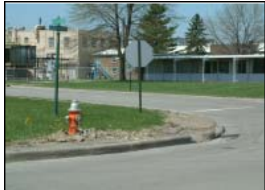
Broken and over-driven curbing with damaged shoulders convey negative images.
