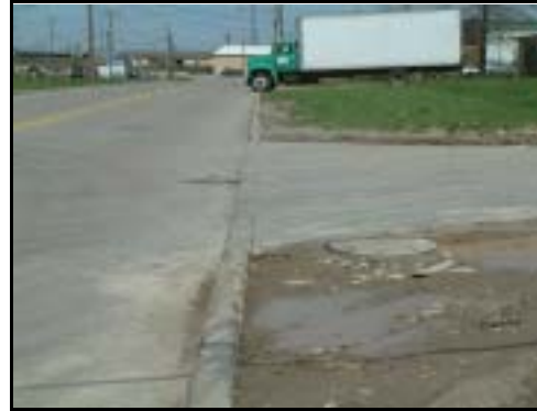
Over-driving of undersized access drive aprons is common throughout the Village's industrial district.
