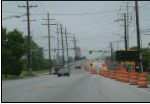
The Northfield Road bridge, a key Village “gateway” underwent major reconstruction during 2004.
