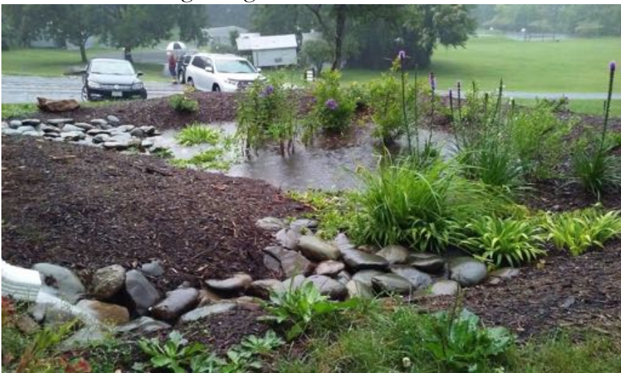
Figure 128. Bioswale (image courtesy of Virginia Association of Soil and Water Conservation Districts, 2019)
