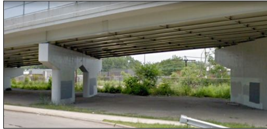
Figure 116. Gramatan Underpass Before
